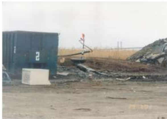
Fig. 7: Methane Gas Vent
