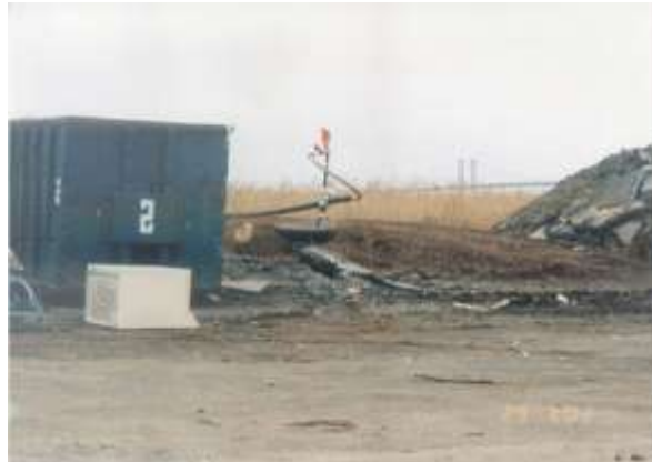
Fig. 7: Methane Gas Vent
